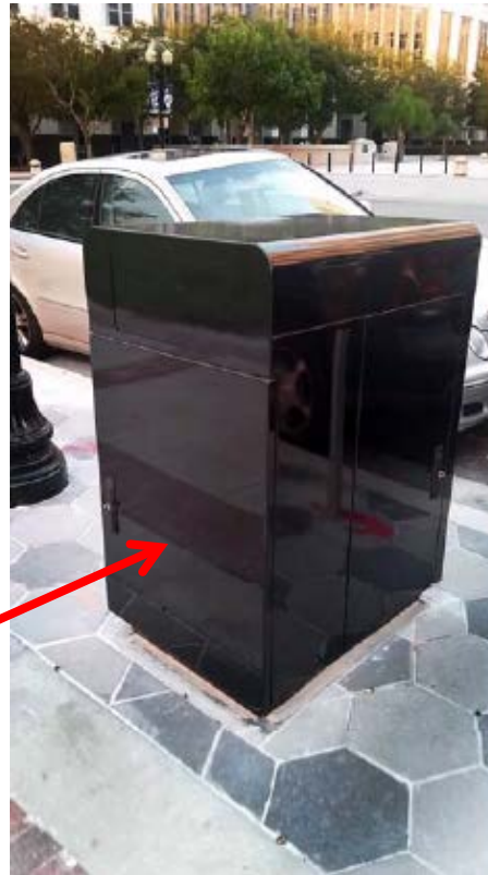
Equipment for Antenna Stored in Functioning Trash Can
